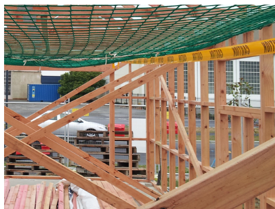
Figure 4: Temporary bracing means that there is not enough clearance below the nets. A person falling onto the net is likely to strike the timber bracing. This is not best practice.
